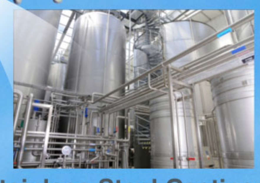
Stainless Steel Casting for Process Equipments
